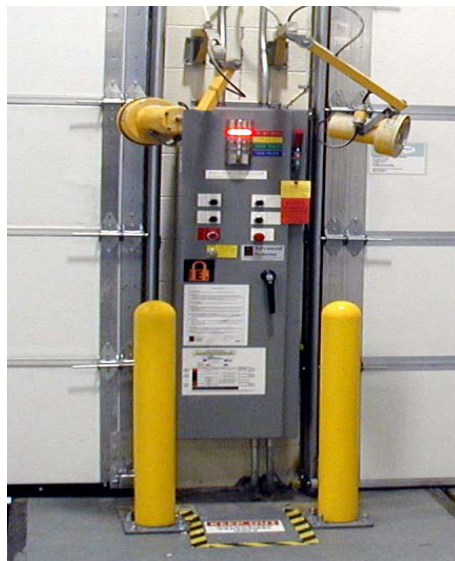
UIDSS CONTROL PANEL
