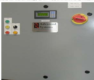
Door Control Panel with Built-in Diagnostics
