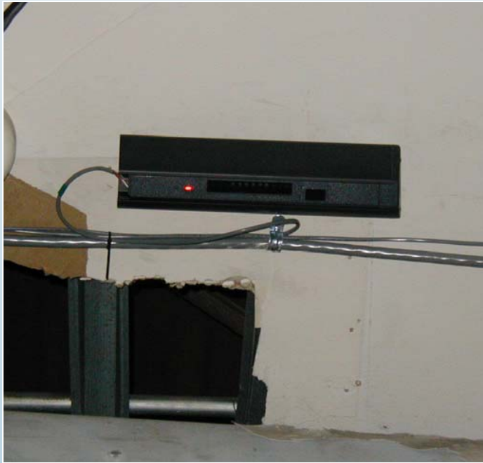
Interior Sensor Monitors Door Area
