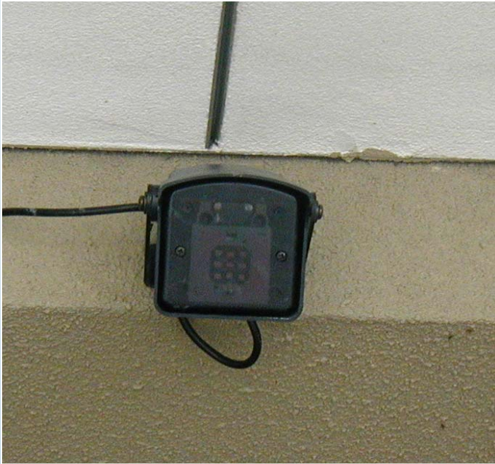
Sensor Notifies Inside Controller of Vehicle Presence
